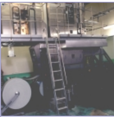
Aseptic Packaging - packaging is performed by the Tetra Brik Aseptic filling machine
